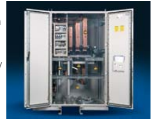
Low voltage switch board
